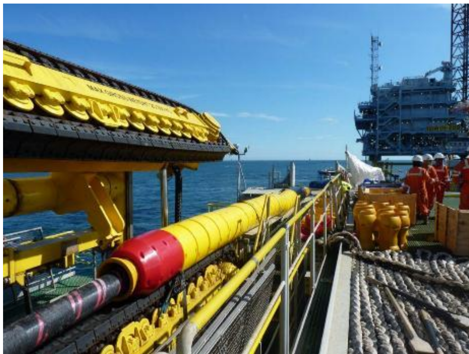
Figure 33 Cable protection system on vessel deck, courtesy of Tekmar.
