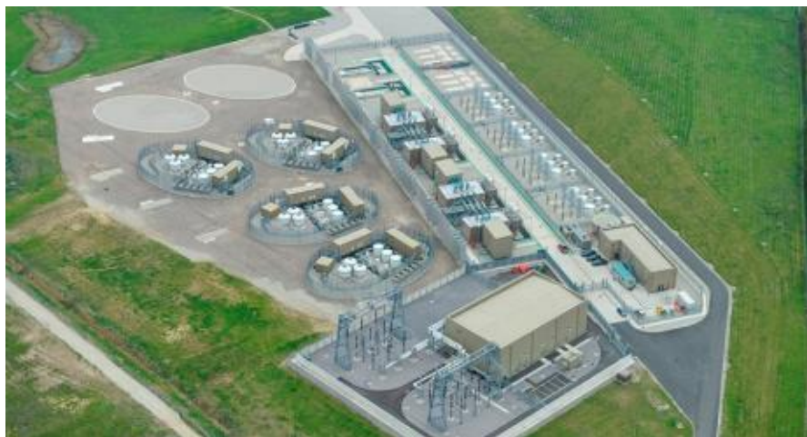
Figure 46 Onshore substation, courtesy of Trant Engineering.
