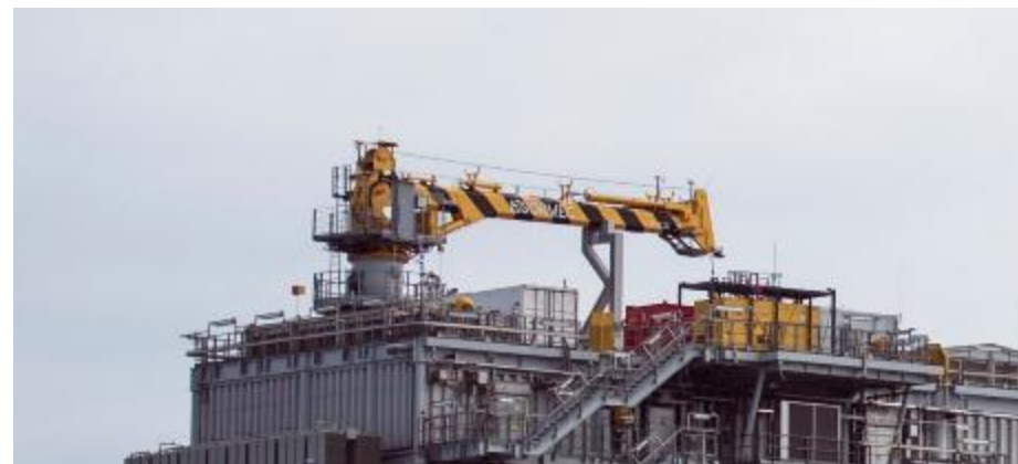
Figure 45 Offshore substation crane and storage facilities, courtesy of Equinor, © Ole Jørgen Bratland.
