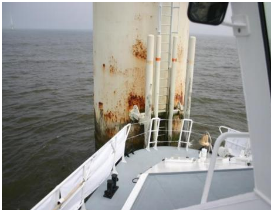
Figure 41 Corroded monopile structure, courtesy of Materialenkennis.
