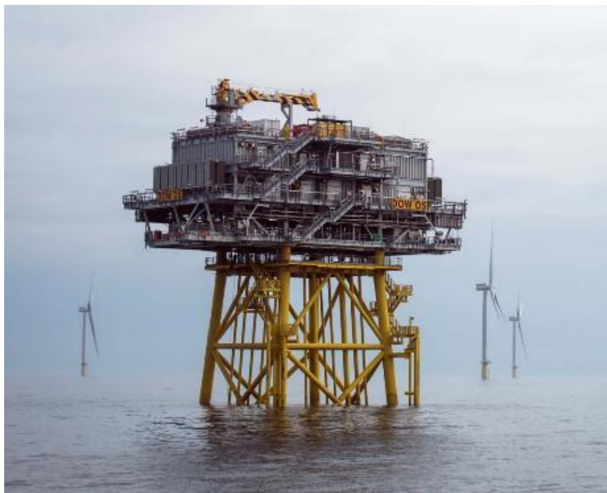
Figure 43 Offshore substation, courtesy of Equinor, © Ole Jørgen Bratland.
